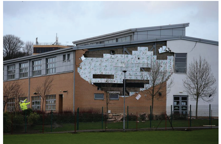
Oxgangs Primary School collapse
